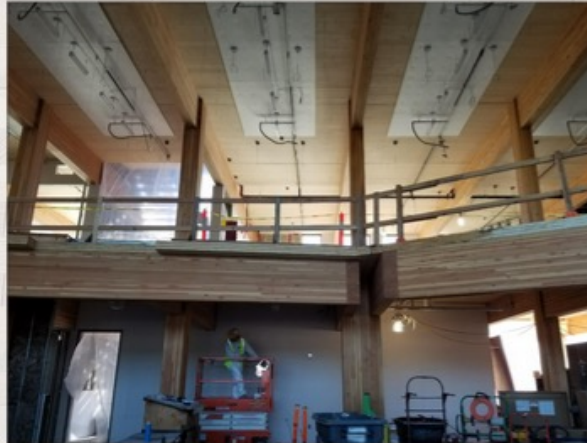
First Tech Credit Union is building its new headquarters in Oregon from CLT manufactured in Canada
